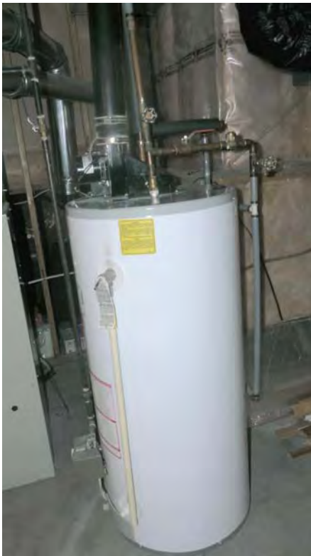
Hot Water Tank, gas hi efficient, Infloor basement heating and domestic hot water
