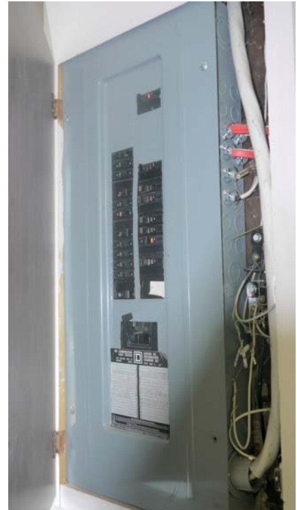
200 amp Breaker Panel
