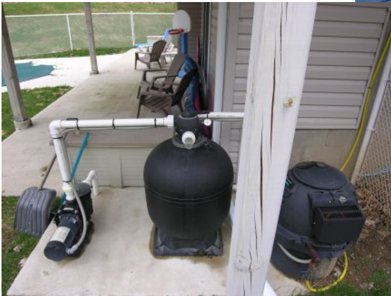
Swimming Pool Equipment
