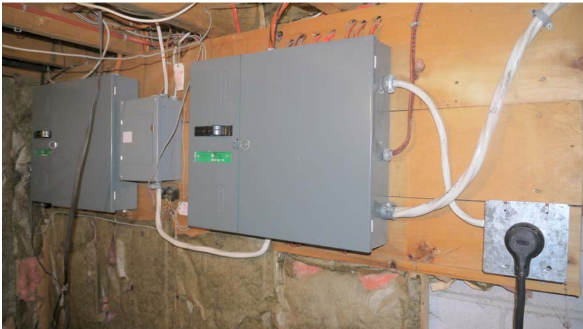
Two 100 Amp Fuse Services
