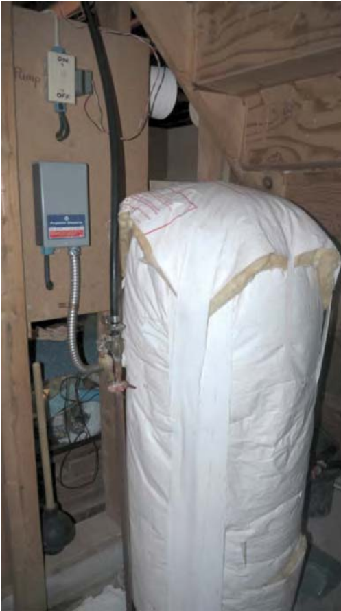
Cold Water Tank
