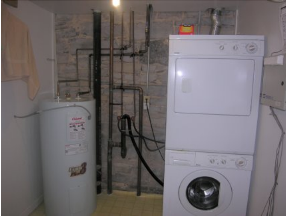
Hot Water Tank
