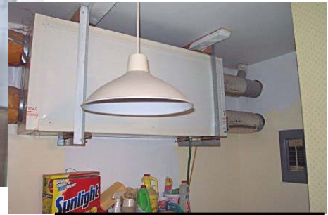
Laundry Room off Kitchen with Air to Air Exchanger
