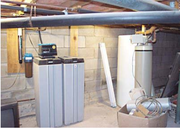
Water Softener and Hot Water Tank
