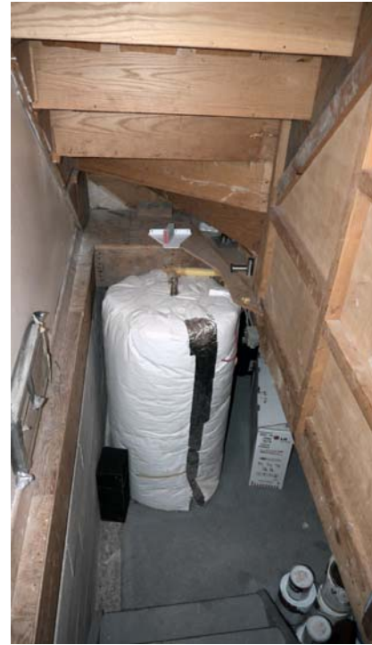
Hot Water Tank
