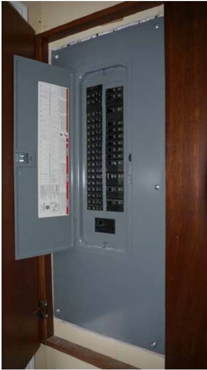
Updated Wiring , Electrical Panel
